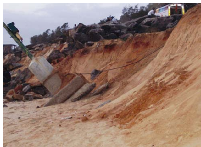
Fig. 3— Severe erosion at Maravanthe beach in Karnataka state of India, threatening NH-17 12 .
