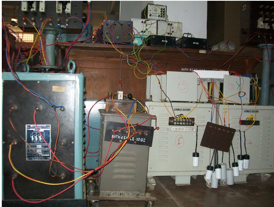
Figure C.2: View-1 of the passive filter
