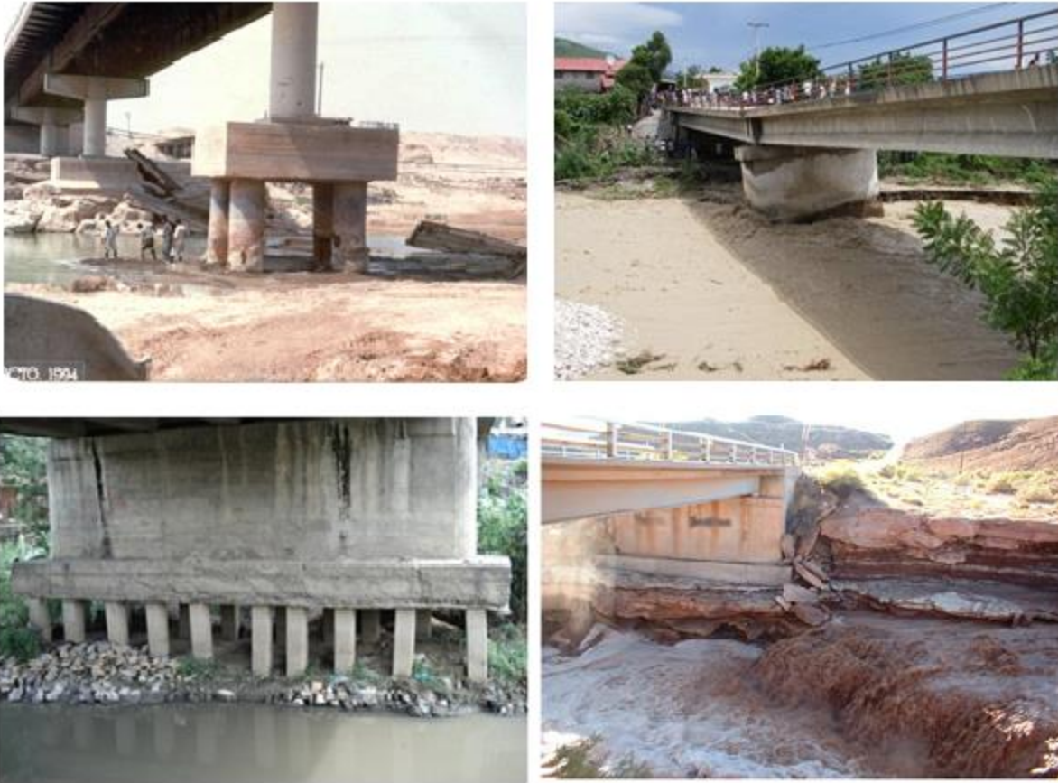
Figure 1.1 Formation of scour around the bridge pier and abutments
