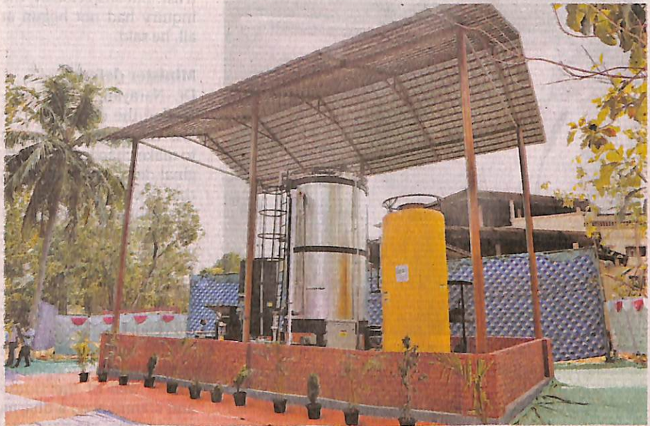
The 500 kg food waste biogas plant installed on the premises of NITK, Surathkal, is in operation. SPECIAL ARRANGEMENT
