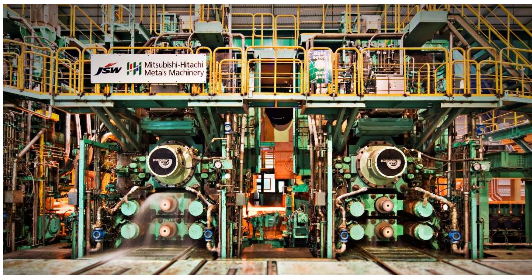
Fig. 5.7. Finishing mill stand controlling strip thickness
