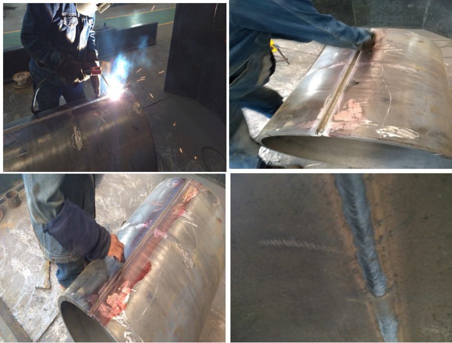
Fig. I.3 Identification of cracks after welding in classifier shell
