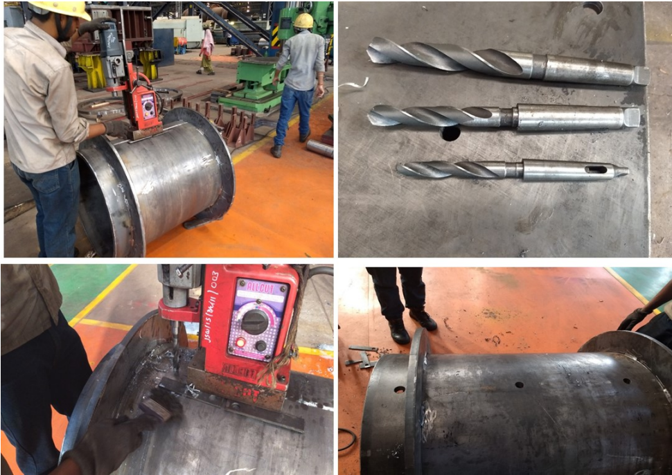
Fig. I.7 Drilling of out let valves in classifier shell by using magnetic drill machine
